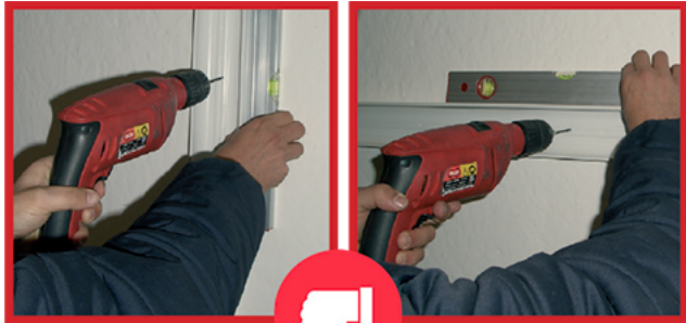
Duct installation without built-in level
