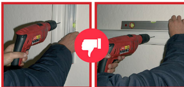
Duct installation without built-in level
