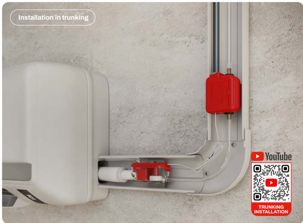
Installation inside the split unit
