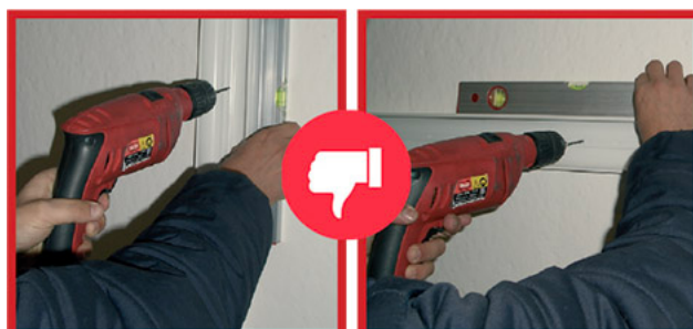
Duct installation without built-in level
